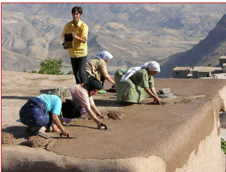
The women of Kazaj village are plastering the facade of a house.
