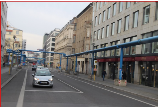
4) What are the blue pipes for and in which city?
